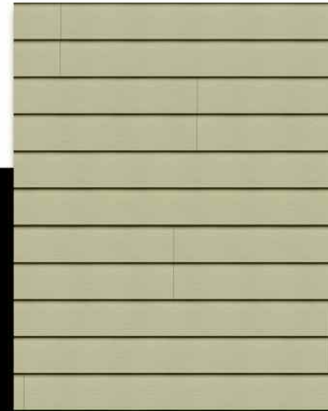
Other Cladding: Double Courses Causing Stacked Seams
